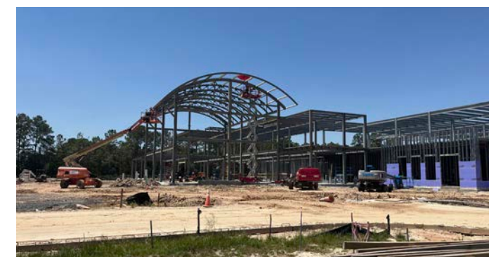
When complete, STHS’s 126,000-square-foot Ambulatory Surgery Center will boast 12 surgical suites and array of support services. Ground was broken in November 2023, and completion is set for summer 2024. (Photo by Mike Scott / STHS)
