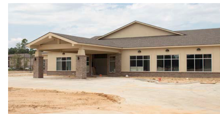
Construction continues apace on a new, 18,000-square-foot family medicine clinic north of Covington. It is expected to be complete in January. (Photo by Tim San Fillippo / STHS)
