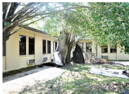
Ida's winds ripped a portion of the roof from the Covington building housing STHS's Express Care walk-in clinic and St. Tammany Pediatrics, which is temporarily operating out of the St. Tammany Physicians Network clinics in Mandeville and Madisonville. (Photo by Mike Scott / STHS)
