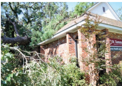
STHS's Home Health and Hospice building was destroyed by a tree during the storm. After working out of a conference room in Ida's immediate aftermath, the operation has since been temporarily relocated to the STHS Palliative Care office at 1010 S. Polk St. (Photo by Melissa Hodgson / STHS)
